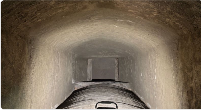
Build-up forming on the lining
