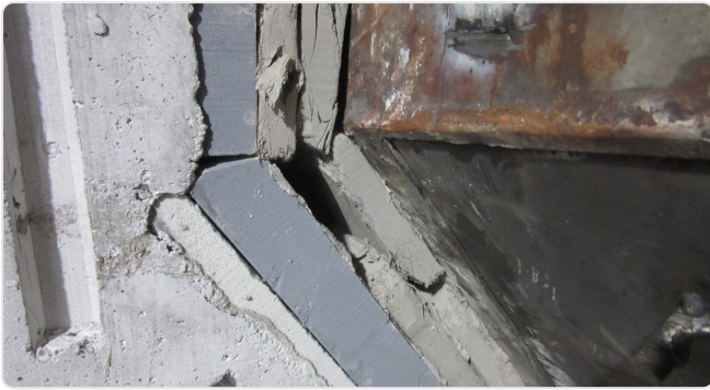
Finding: the lining is cracked right down to the steel shell
