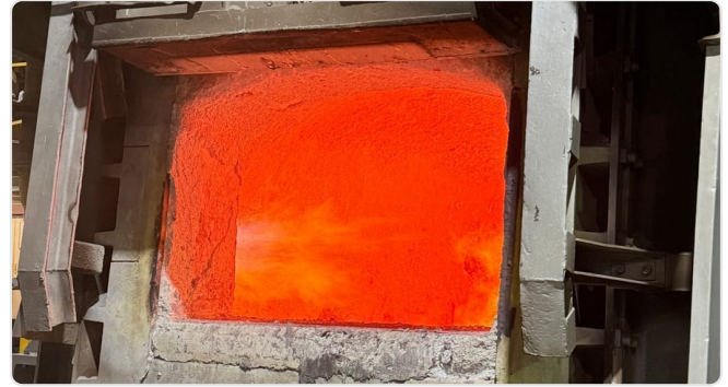
Glowing lining in operation
