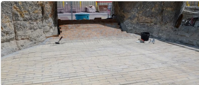
Freshly lined furnace section before the controlled heat-up
