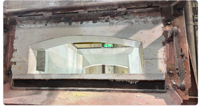
Furnace front: opening and door fit the new geometry
