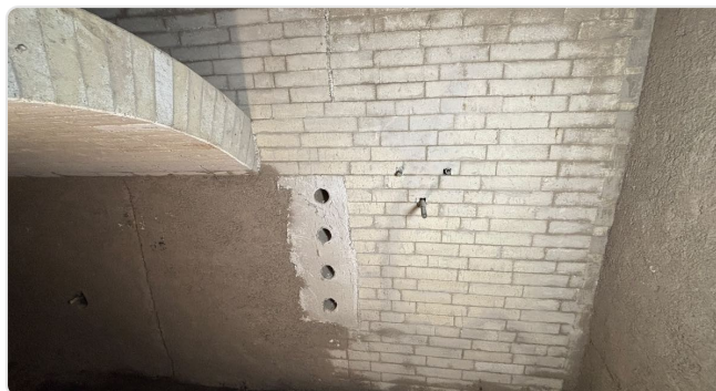
Secondary air openings set during installation
